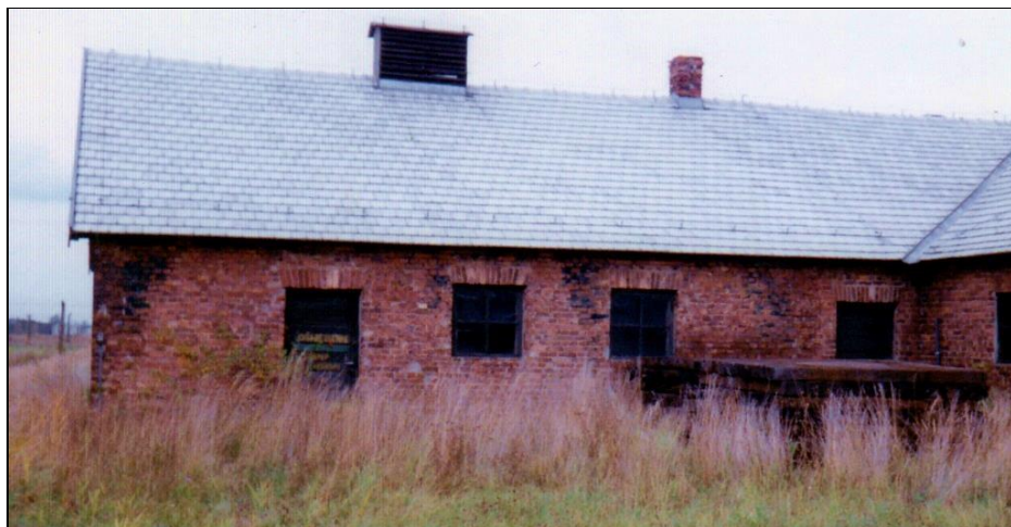
Figure 168: Disinfestation wing of Building 5b, southern wall (of Rooms 4 and 5 in Figure 40) with some staining. (© C. Mattogno 1991)
