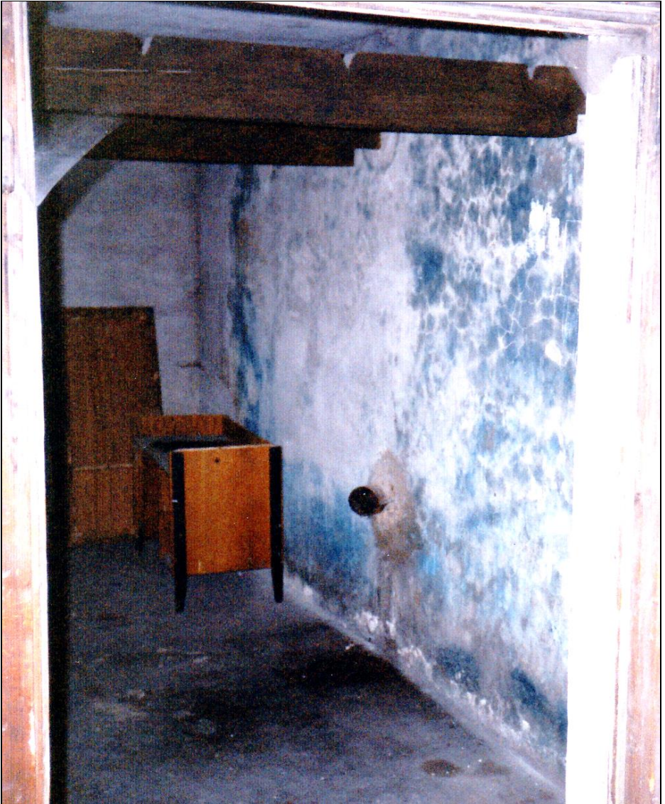
Figure 159: Disinfestation wing of Building 5a, eastern internal wall seen from the south, not quite as intensely stained as external walls (Room 1 in Figure 40, seen from the south). (© C. Mattogno 1991)
