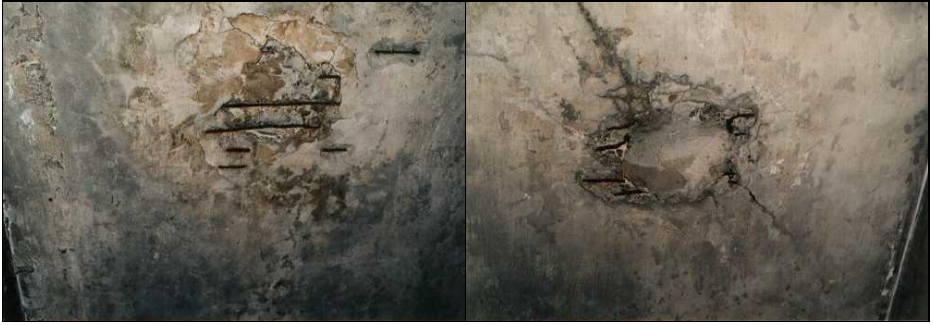
Figures 52 and 53: Two of the four former openings through the flat roof of the morgue of Crematorium I in Auschwitz Main Camp, visible at the ceiling. They probably served as ventilation openings for the air-raid shelter in 1944. They were closed after the war “for museum purposes,” because their location makes it obvious that they couldn’t have served as Zyklon-B-introduction holes.
