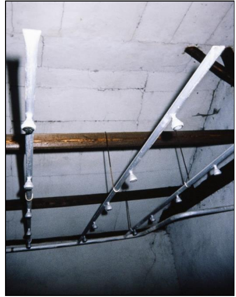
Figure 43: Water-pipe system with shower heads in the disinfestation wing of building BW 5b. These water pipes have no connection; they terminate in the ventilation outlets. See Figure 42.
