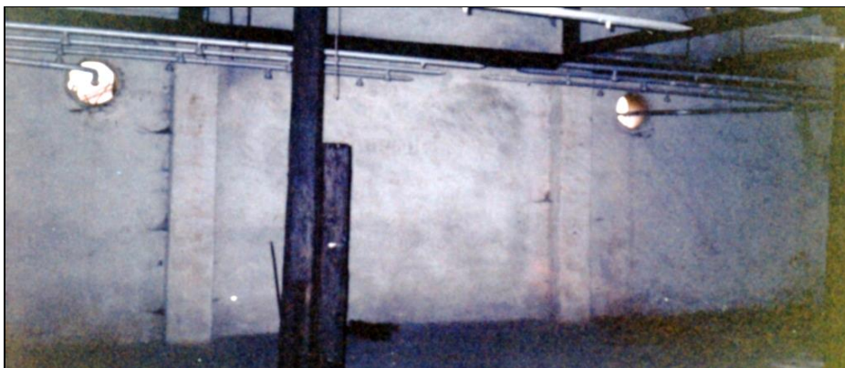
Figure 149: East wall of the delousing wing of Building BW 5b with only minor stains on the plaster rich in lime and poor in iron.
