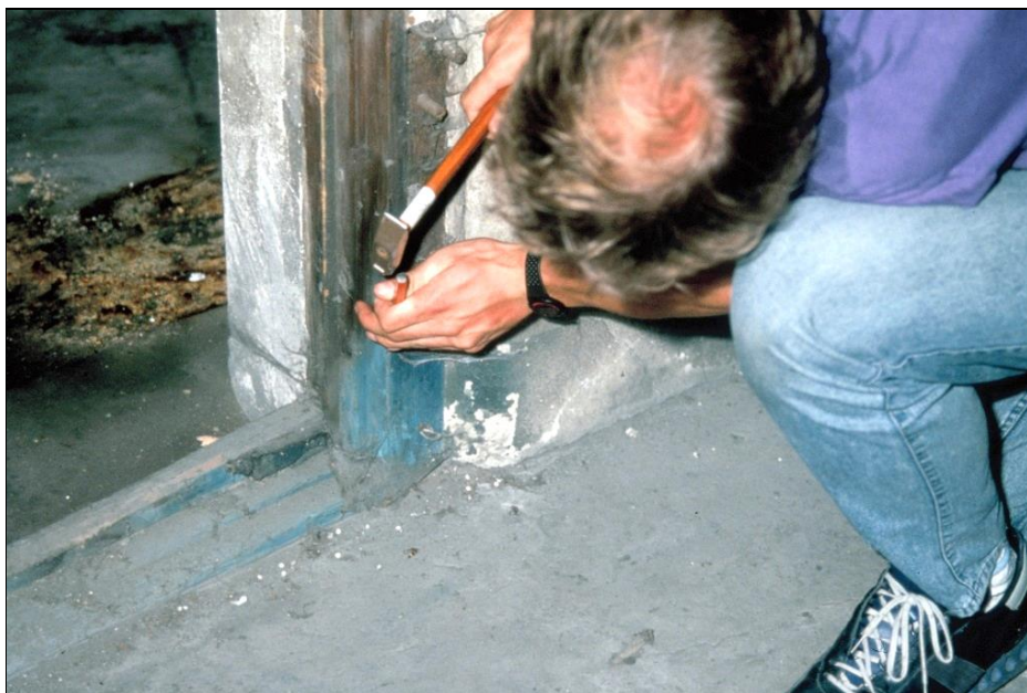
Figure 148: Picture of the door frame in disinfestation wing of Building 5a (between Room 2 and Room 1 in Figure 40) with the author. The lower, rusty hinge has developed Iron Blue under the influence of hydrogen cyanide. Sampling location of Sample No. 18.
