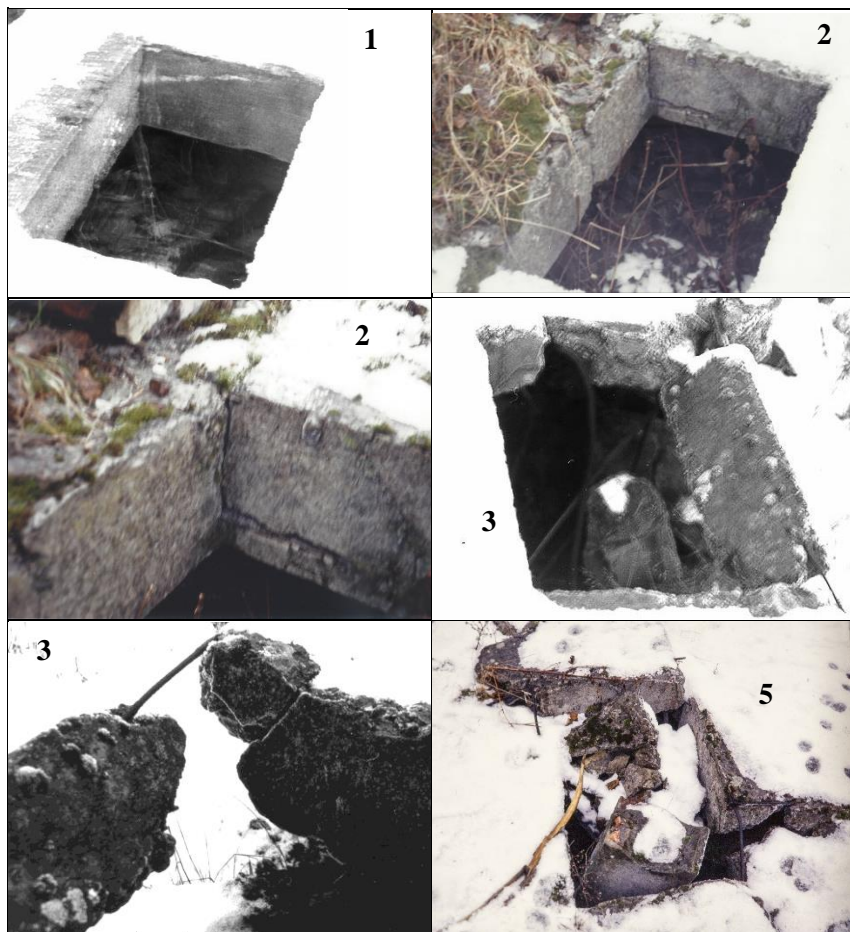
Figures 91-96: Four of the five properly constructed ventilation holes in the ceiling of the furnace room on the ground floor, Crematorium III (no. of holes indicated; #2 and #3 twice); condition: December 18, 1991. Note the cracks caused by the explosion, especially at the corners. The close-up photo of Hole #3 (third row on the left) shows a reinforcement bar running around the hole and still holding the concrete fragments together.
