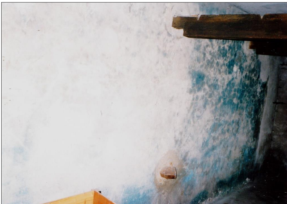
Figure 158: Disinfestation wing of Building 5a, eastern internal wall seen from the north, intensely stained only along the floor and in the southern section (Room 1 in Figure 40). (© C. Mattogno 1992)
