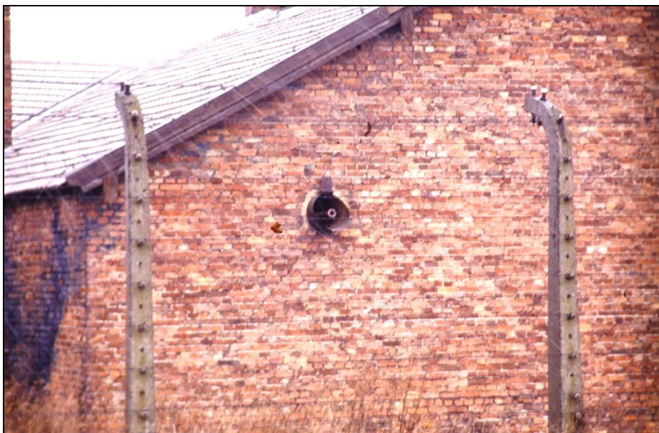
Figure 42: Ventilation outlets from the disinfestation wing of Building 5b, without equipment today. The ends of the water pipes are visible inside; see also Figure 43.
