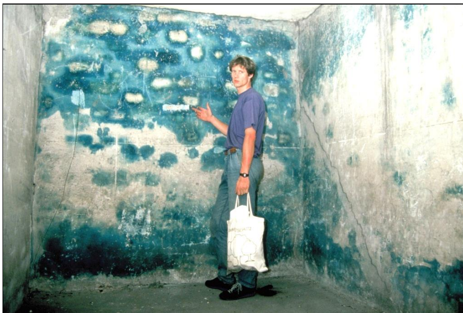
Figure 146: Room located in the northwest of the disinfestation wing of Building 5a (Room 4 in Figure 40) with the author. The exterior walls are located in the background and to the right, showing intensive blue discolorations caused by Iron Blue. Sampling locations of Samples 9 and 11 are visible. On the left in the picture is the interior wall, erected during the conversion to a hot-air-disinfestation chamber. Sample 10, with a slightly positive cyanide content, was taken from this wall.
