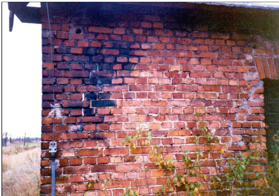
Figure 169: Disinfestation wing of Building 5b, southern wall, with some staining at the corner. (© C. Mattogno 1991)
