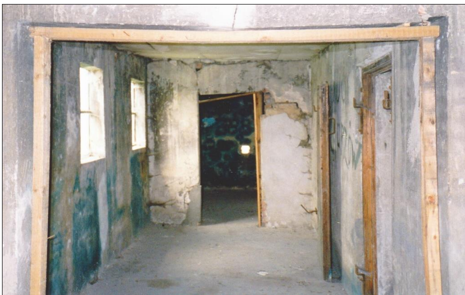
Figure 153: Disinfestation wing of Building 5a, with the southern external wall on the left. Look through Room 2 into Room 3 in the background (see Figure 40). (© C. Mattogno 1992)
